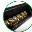
Neutral & Grounding Terminal
