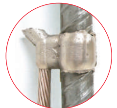
• 95 mm 2 Copper Cable to 40mm Rebar
